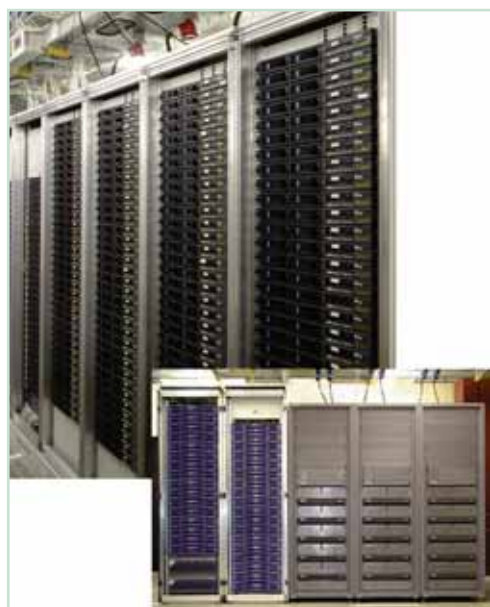
Fig. 3: A part of the CeBiTec compute cluster and storage systems including 128 SunFire V20z dual Opteron servers and several Sun StorEdge 351x and A3500FC cabinets.
